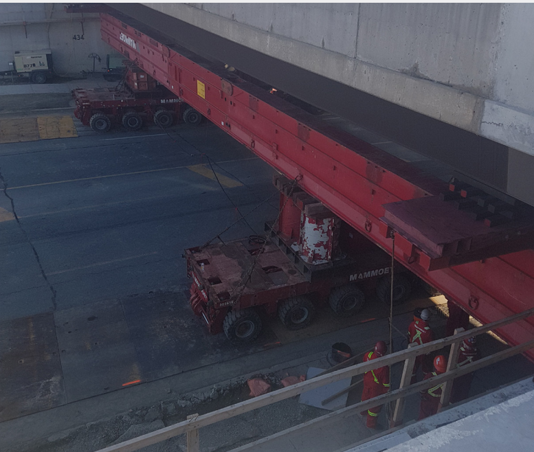
View from Albion Road of Self-Propelled Modular Transporter machine set up below Albion Bridge on Saturday June 16 prepared for the bridge move.
