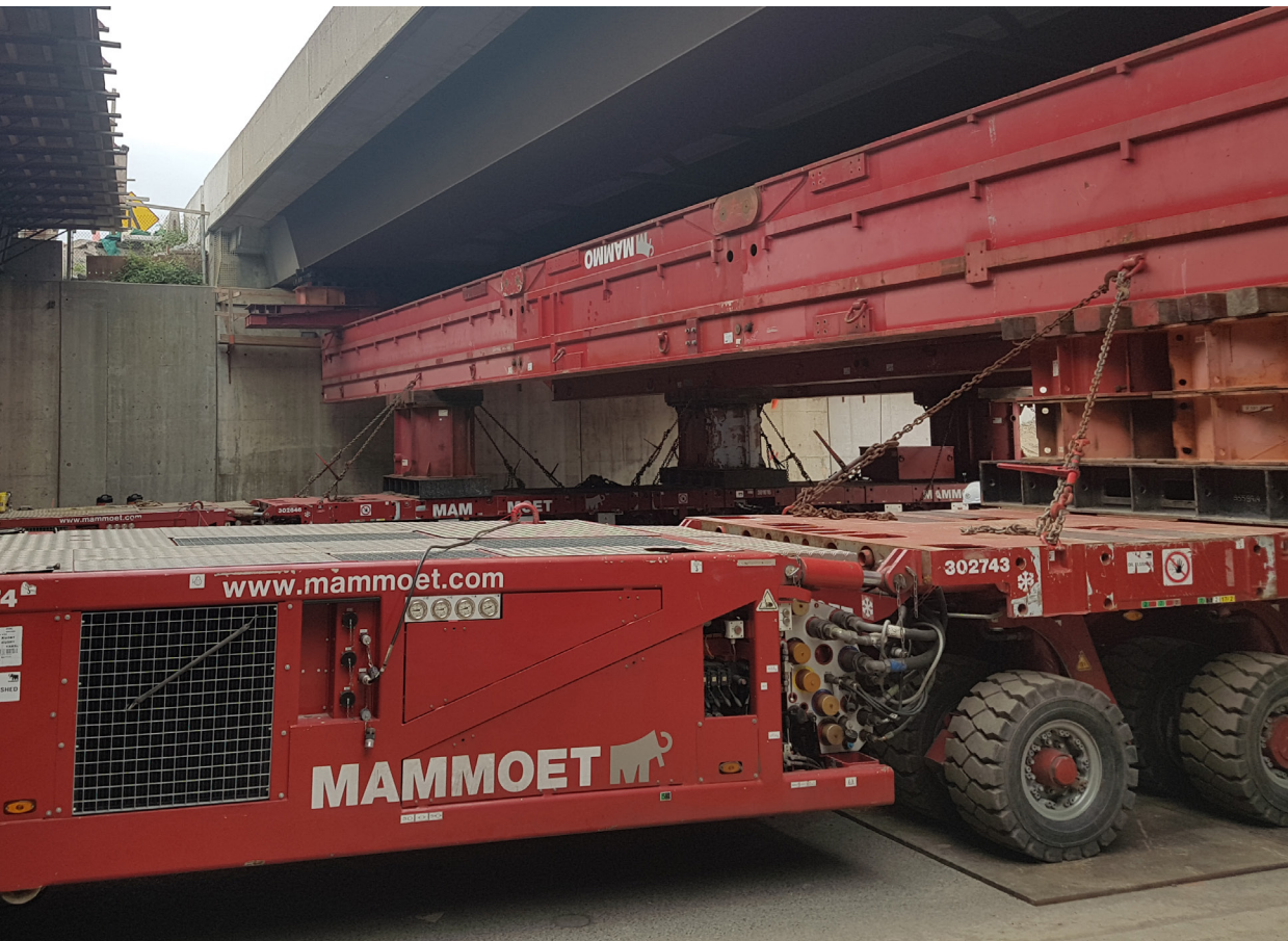
Close up view from Hwy 427 of Self-Propelled Modular Transporter machine set up below Albion Bridge on Saturday June 16 prepared for the bridge move.
