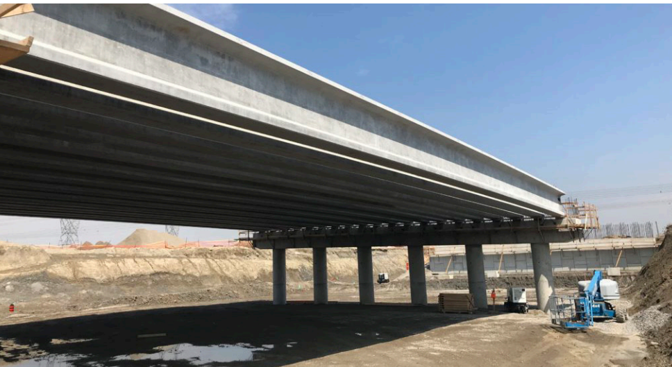
Girders installed at Langstaff Road. The girder is called an I-beam structure because the beam is shaped like an I.
