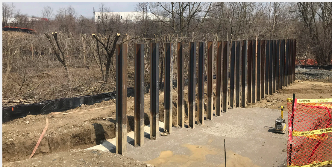
A photo of piles for a deep bridge foundation at Rainbow Creek.
