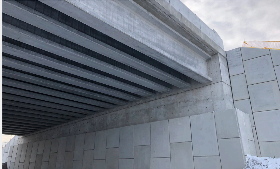
An abutment and RSS walls at the Langstaff Road bridge over Highway 427. The bridge's girders and deck (the superstructure) are installed along the top edge of the abutment.
