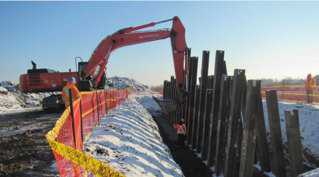
A photo of piles for a deep bridge foundation that were installed in January 2019.
