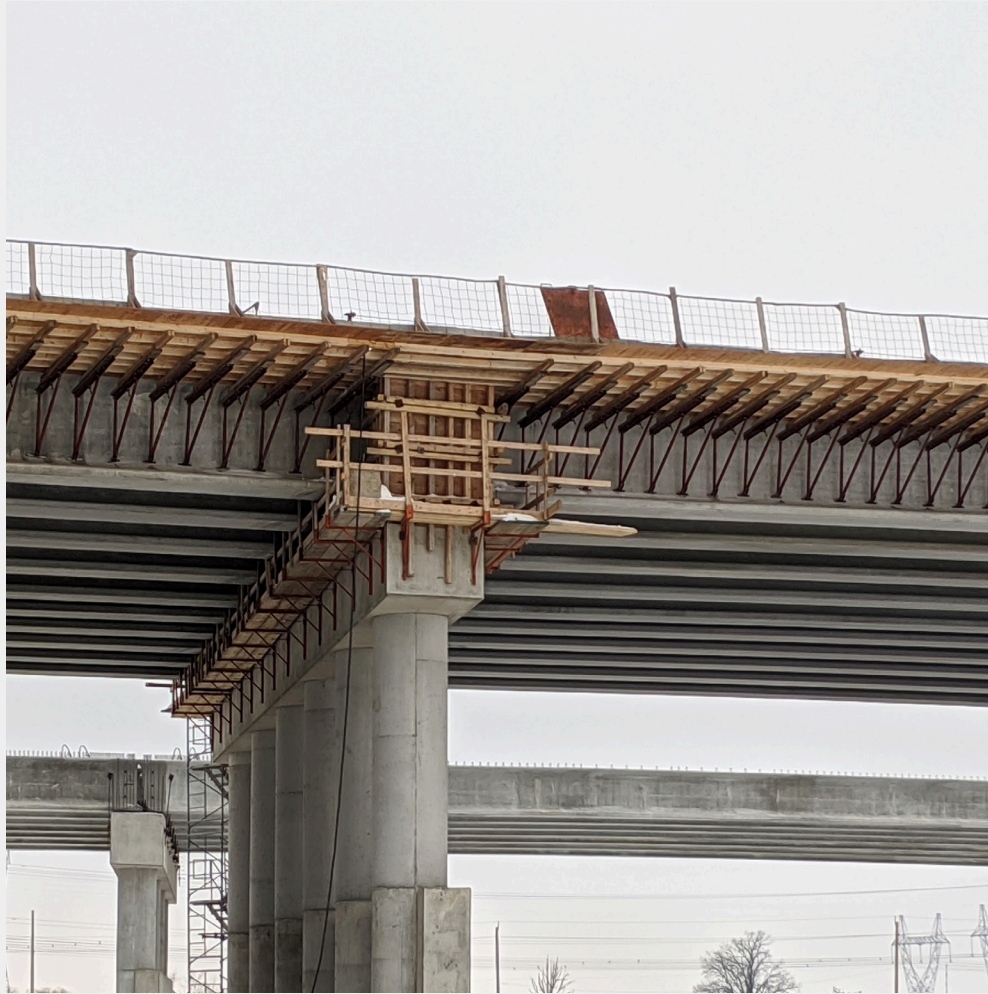
A view of the wooden forms that are being built on the girders to allow for the pouring of a concrete deck over the CP Rail tracks.
