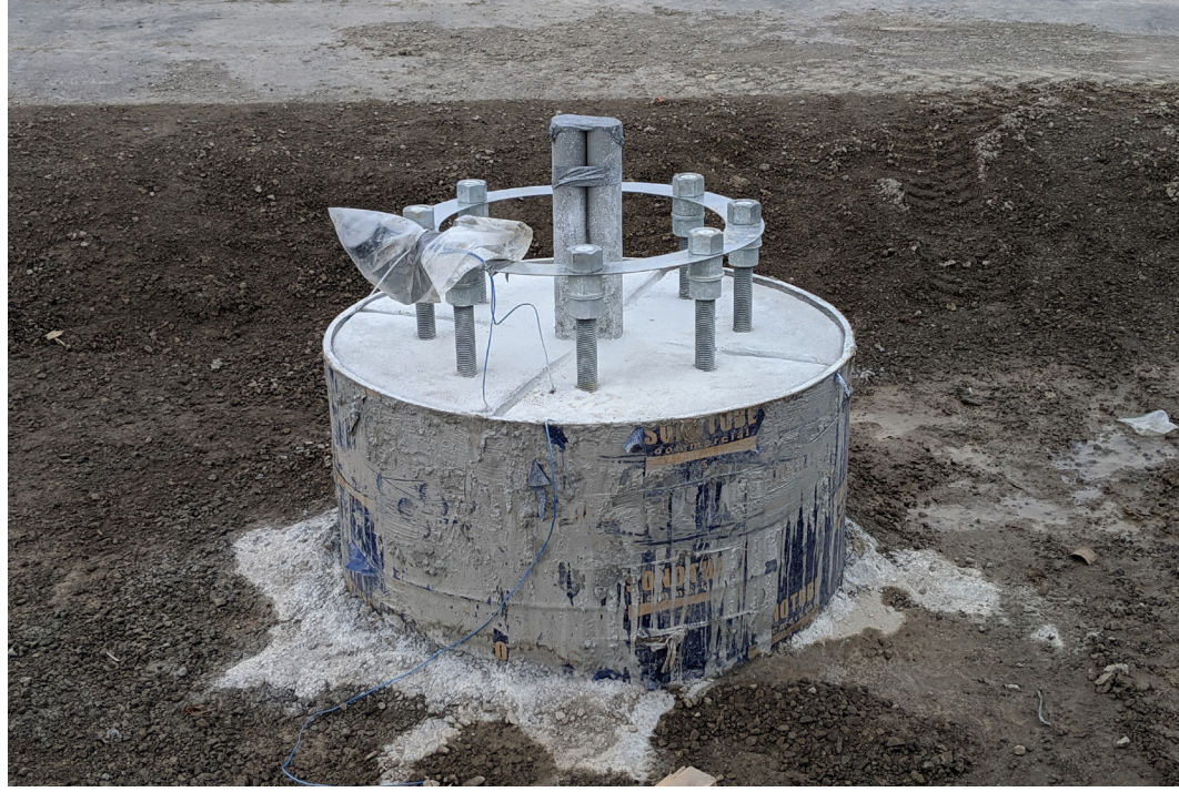
Anchor bolt assembly for a high-mast light pole.
