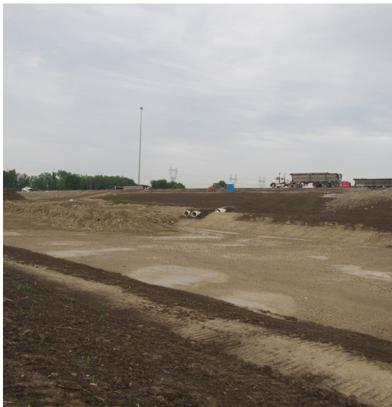
A dry pond being constructed along the Highway 427 Expansion south of Rutherford Road.
