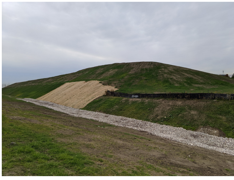
Vegetated embankment and ditch being finalized between Zenway Boulevard and Langstaff Road.
