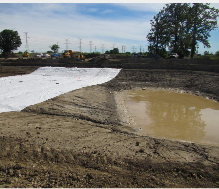
A wet pond being constructed and lined near the Highway 407 ETR interchange.
